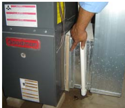
Furnace Filter Location
