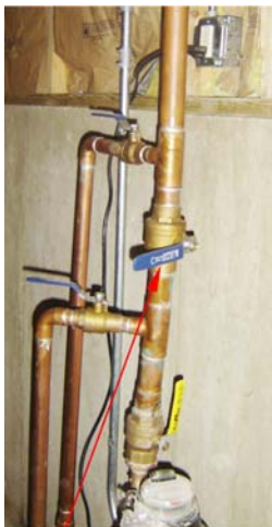
Main Water Shut off Valve
