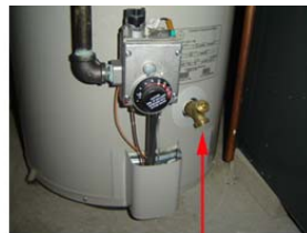
Water Heater Drain Valve
