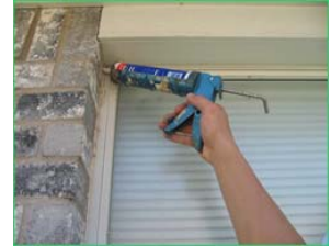
Caulk around windows
