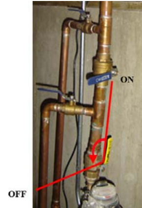
Main Water Shutoff Valve
