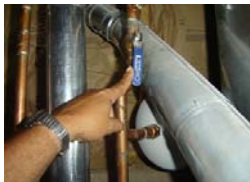
Water Heater Shut off Valve
