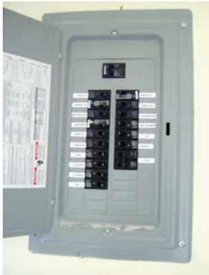
Main Electrical Panel
