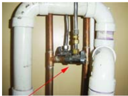
Kitchen Sink Shut off Valve
