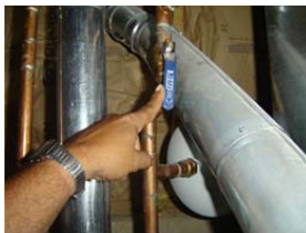
Water Heater Shut off Valve
